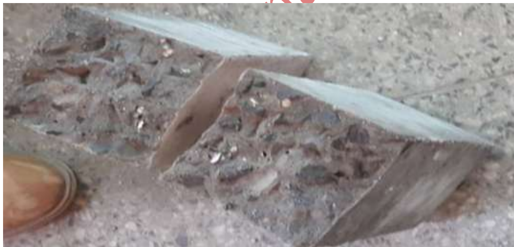
Fig 11: Cracking of uncoated concrete
