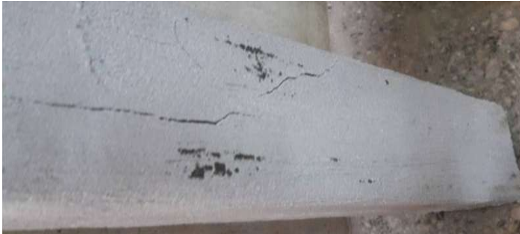
Fig 10: Cracking of carbon fabric coated concrete
