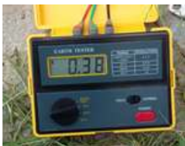
Figure 18 Ground resistance measurement using Earth Resistance Tester
