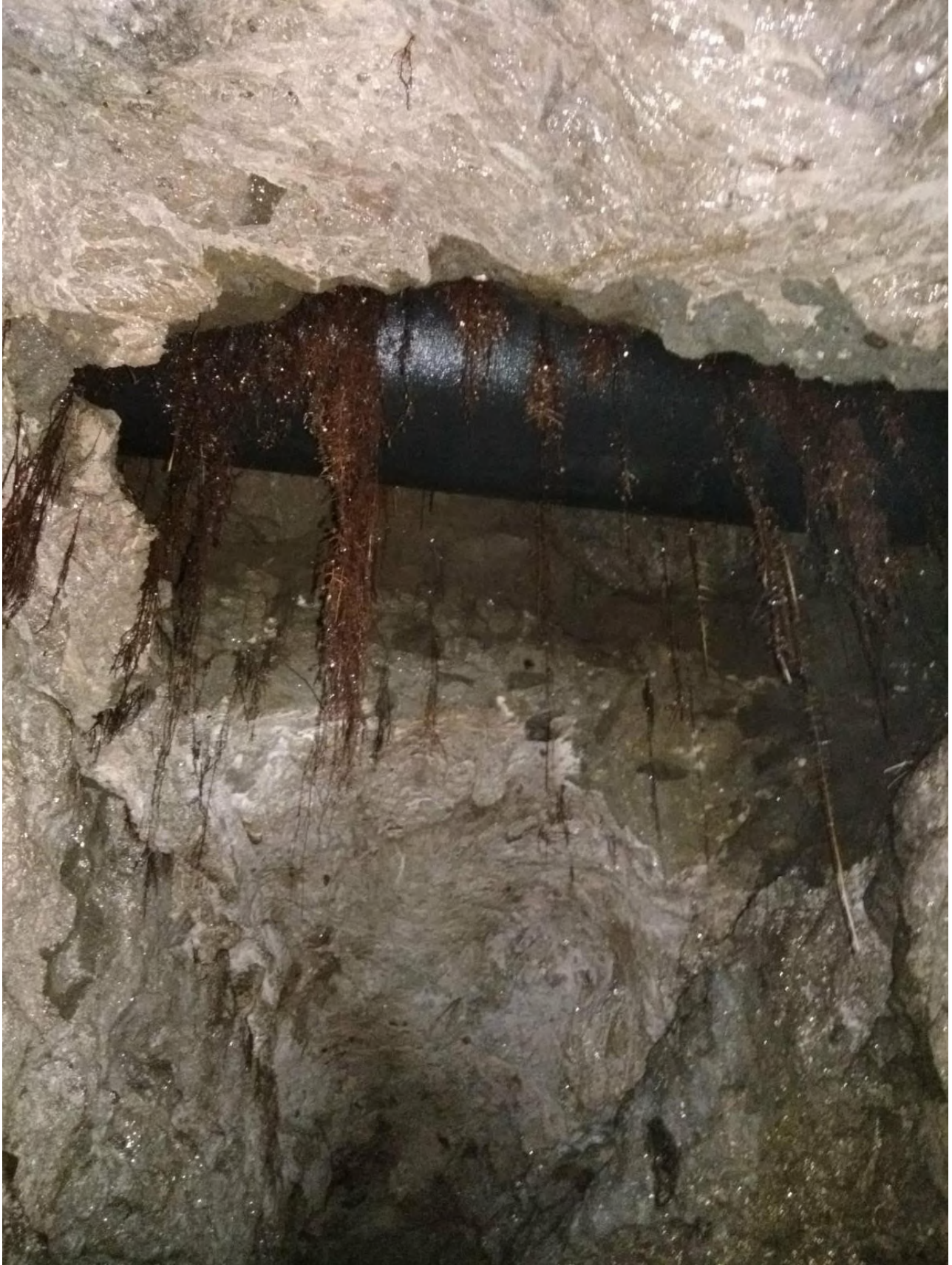
Fig. 5 – Photographic shots inside the ancient and underground conduit. Pipes located just below the road surface can be seen. This proves that part of the ancient conduit was already known. Credits: Giancarlo Valle; Arco di Diana APS.
