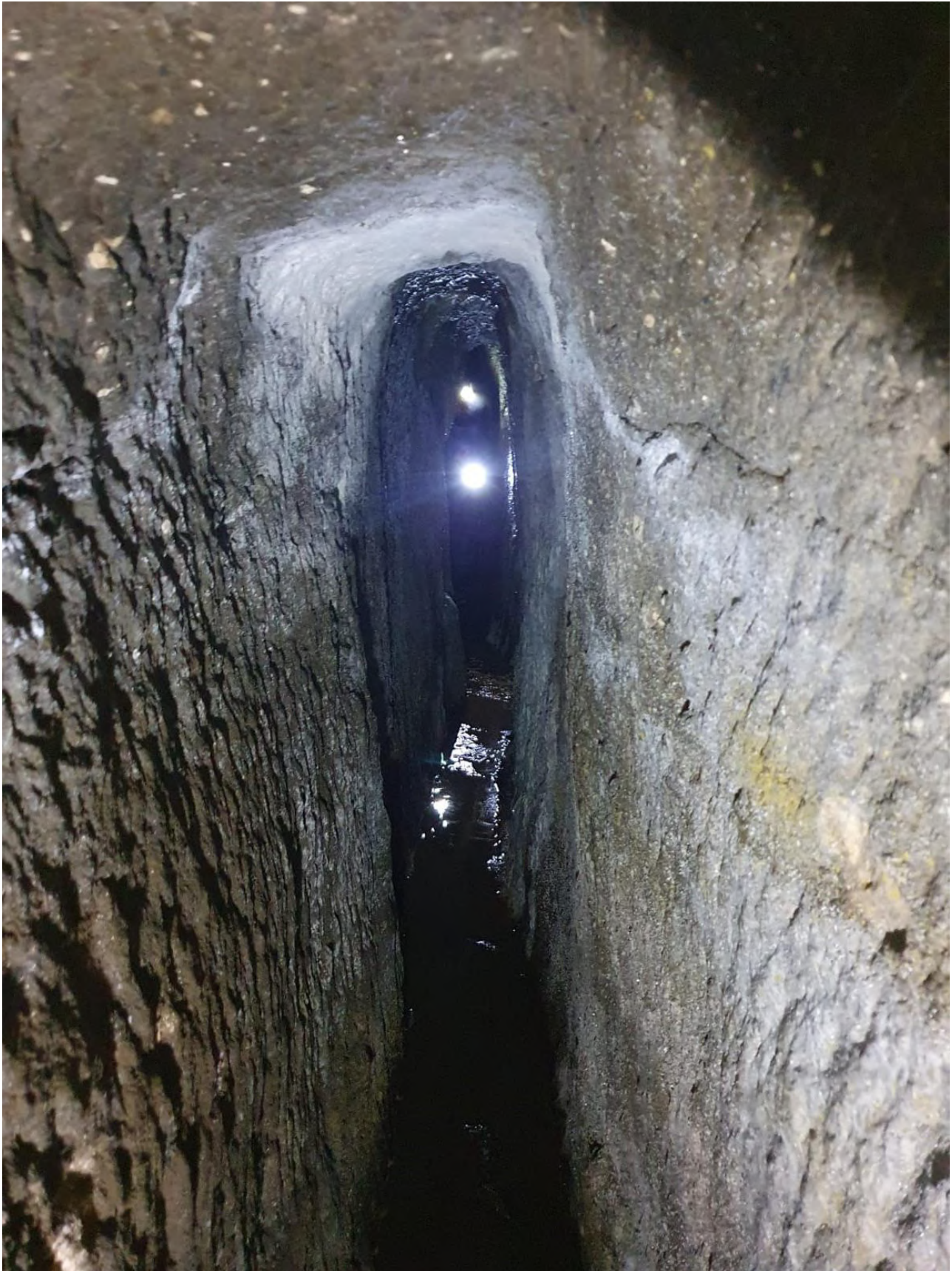
Fig. 7 – Photographic shots inside the ancient and underground conduit. The Arco di Diana APS association (Marco Tudini, Giancarlo Valle, Settimio Tersigni and Riccardo Bellucci), explores the ancient tunnel. Credits: Giancarlo Valle; Arco di Diana APS.
