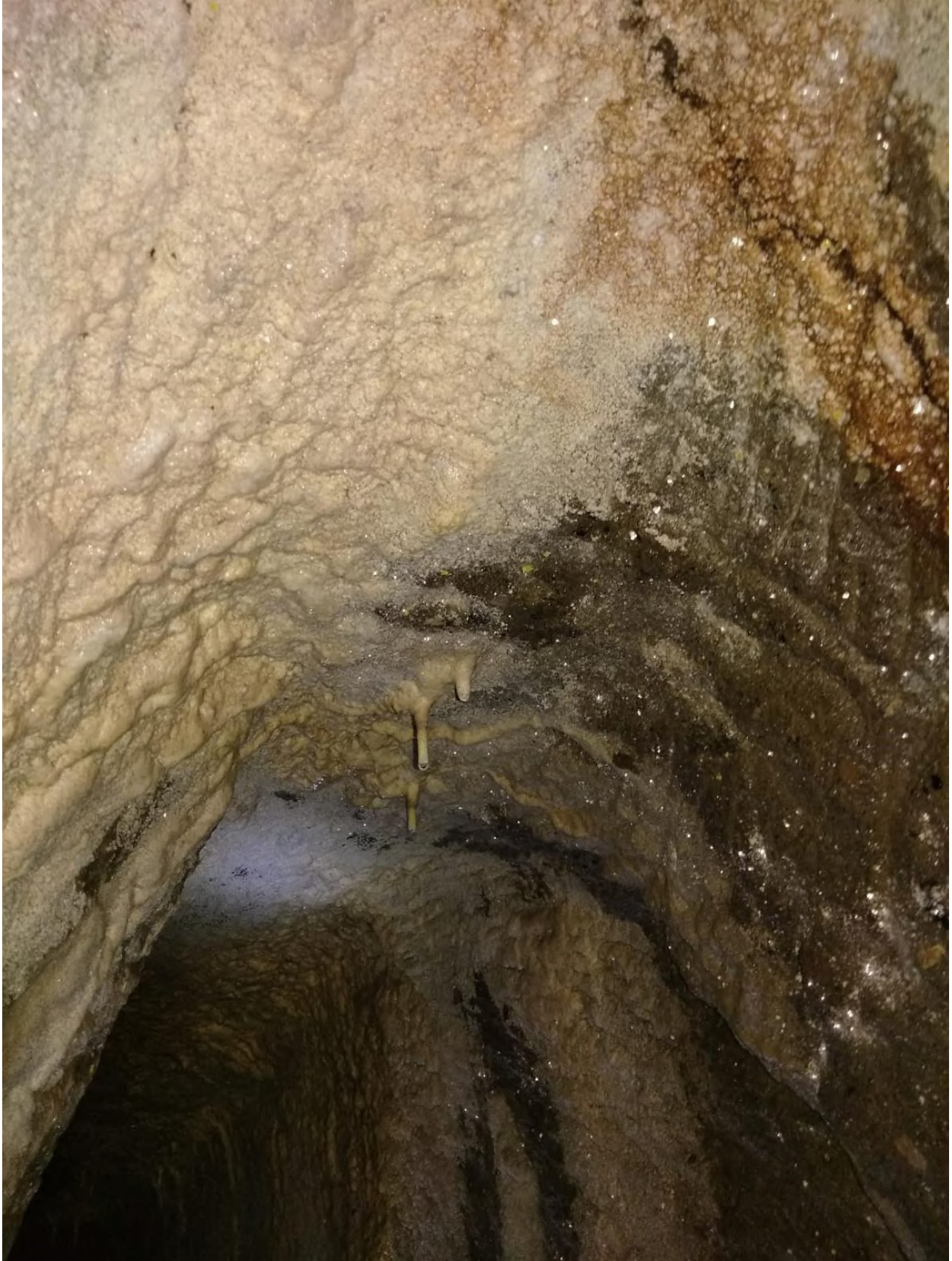
Fig. 12 – Photographic shots inside the ancient and underground conduit. The Arco di Diana APS association (Marco Tudini, Giancarlo Valle, Settimio Tersigni and Riccardo Bellucci), explores the ancient tunnel. Credits: Giancarlo Valle; Arco di Diana APS.
