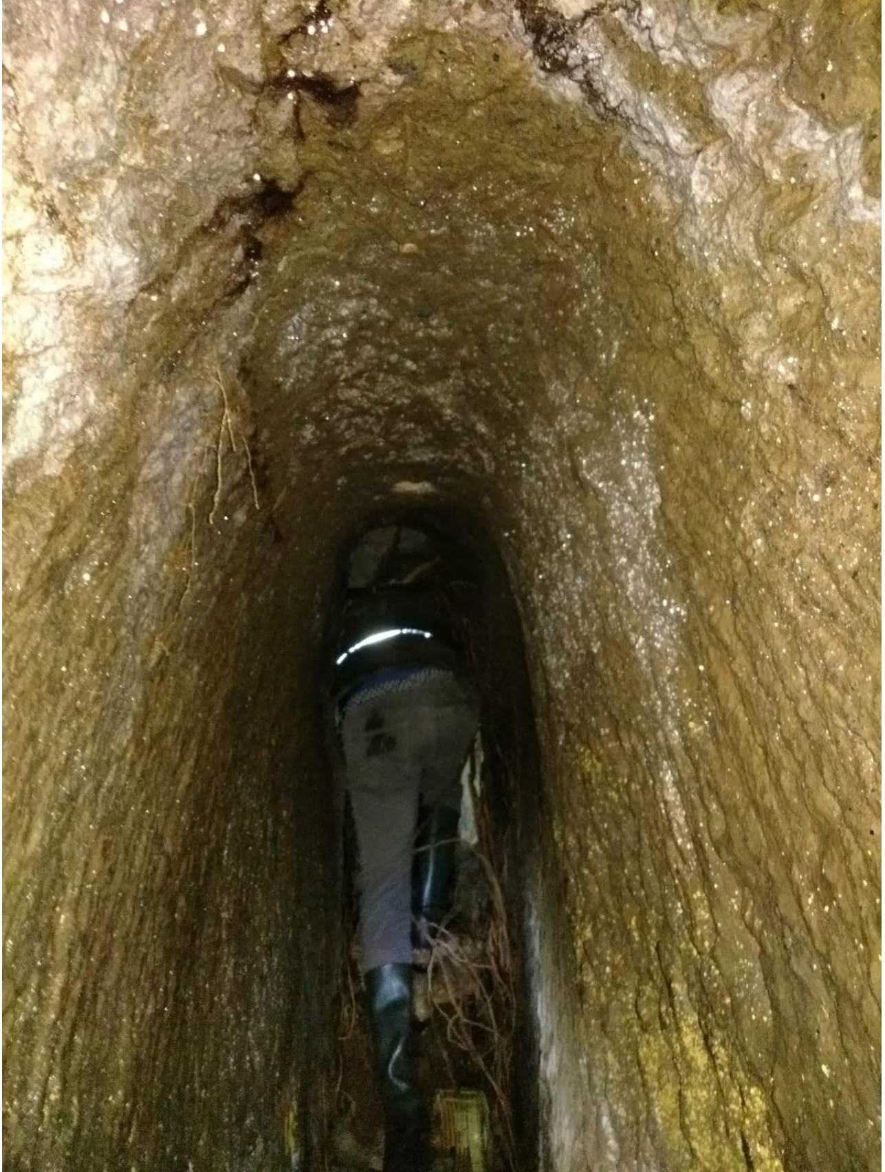
Fig. 4 – Photographic shots inside the ancient and underground conduit. Credits: Giancarlo Valle; Arco di Diana APS.
