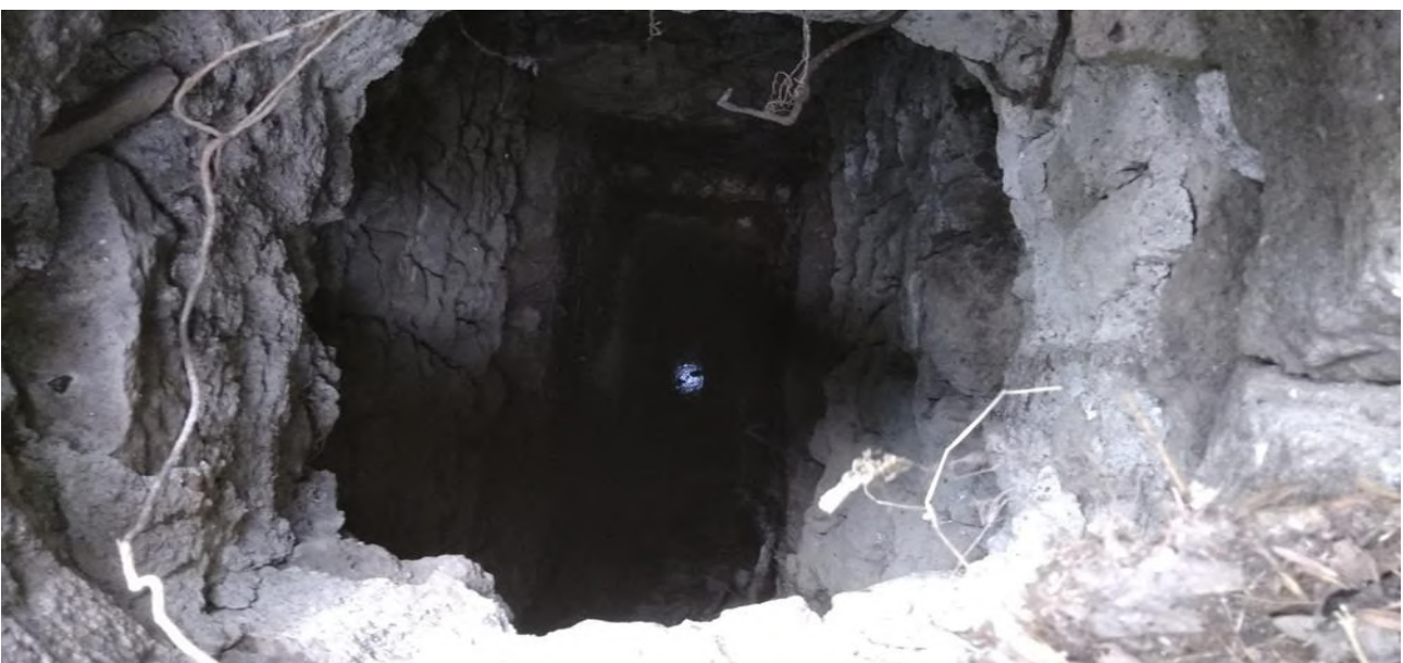
Fig. 20 – Photo of 9 September 2021, taken from the surface of the ground where the accesses to the wells open. In this case, the depth of the well that reaches the ancient underground conduit is documented. Credits: Arco di Diana
